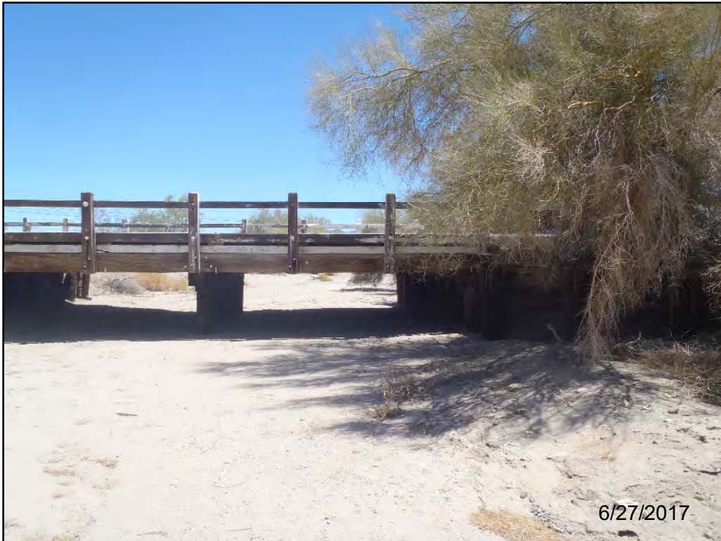
Photo 5. View southwest of Tarantula Ditch Bridge (#56C0103) and the desert wash under the existing timber bridge.
