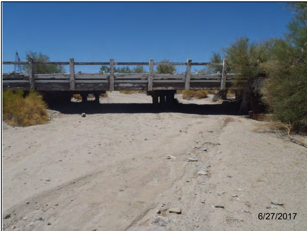
Photo 1. View southwest of timber Aztec Ditch Bridge (#56C0102) and the desert wash.
