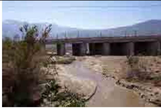
Figure 83. Looking south toward the San Jacinto Mountains at the railroad bridge over the main channel of the San Gorgonio River.
