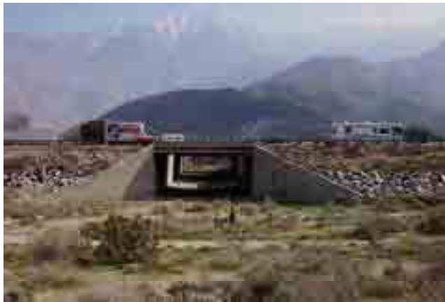
Figure 73. Looking toward the San Jacintos at the westernmost bridges over Stubbe Canyon.
