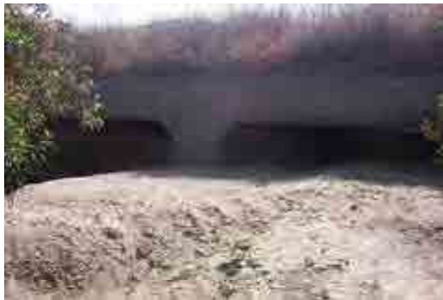
Figure 80. Concrete box culvert under Highway 79, which is in need of maintenance.
