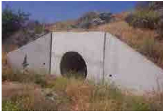
Figure 79. Concrete pipe culvert under Highway 79, which is representative of most culverts along this highway.
