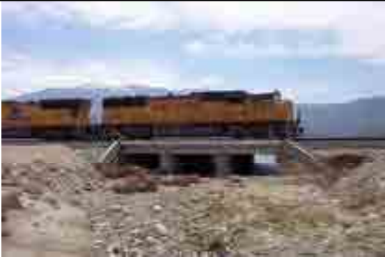
Figure 82. Box culvert built to accommodate overflow of the San Gorgonio River, just west of the bridge to the right. Another similar structure occurs to the east of the bridge.
