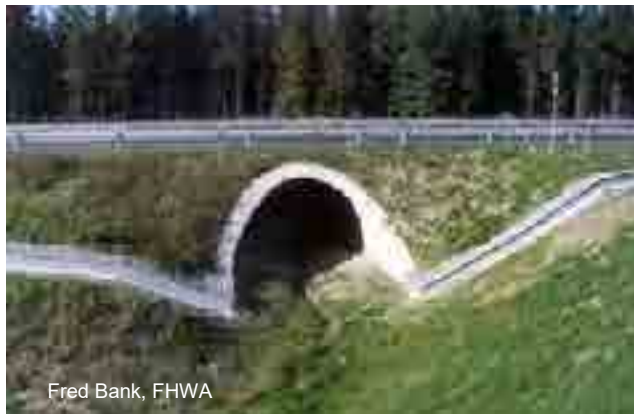
Figure 66. Culvert on German highway, with rail for amphibians and fence for larger animals.
