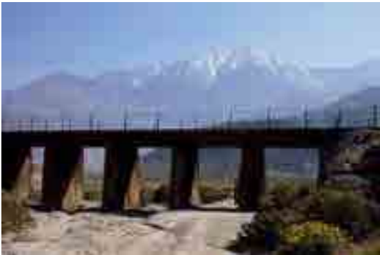
Figure 84. Old railroad bridge over Stubbe Canyon Wash looking toward the San Jacinto Mountains.
