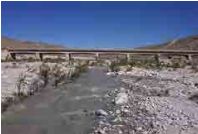
Figure 76. Looking up Whitewater River through the bridge built to accommodate the 2-lane service road.
