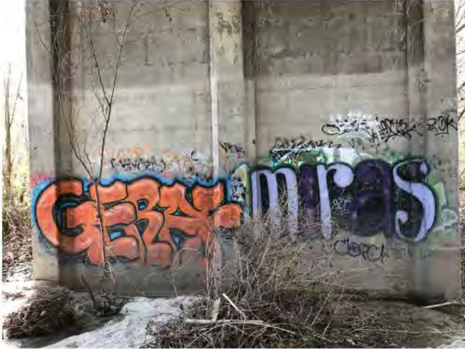
Photo 09: Representative graffiti, Pier 8 facing south (XRF Samples: 028 and 029).
