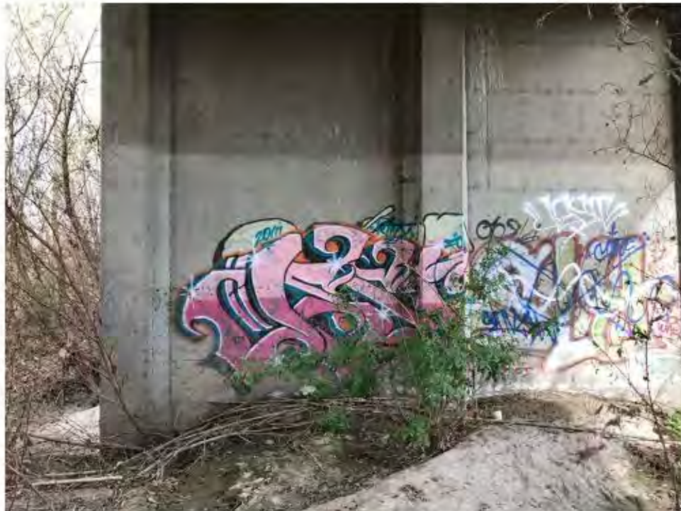
Photo 10: Representative graffiti, Pier 7 facing north (XRF Samples: 030 and 031).
