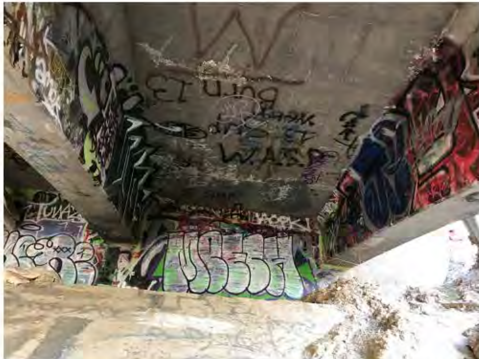
Photo 08: Representative graffiti, South Abutment (XRF Samples: 011, 013 through 016 and 019 through 021).
