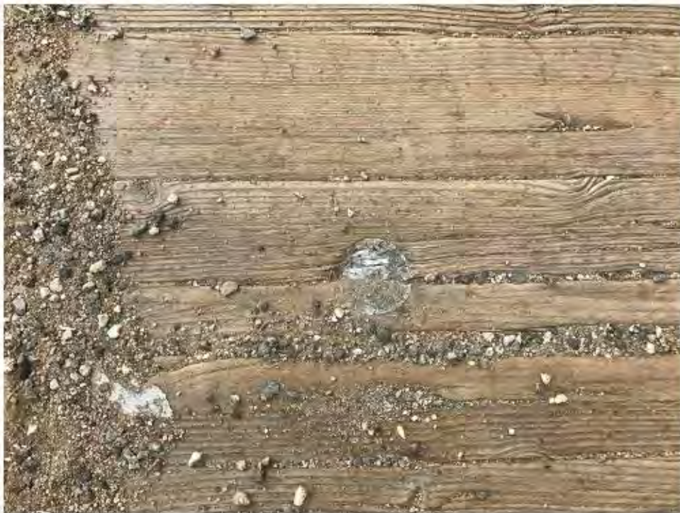
Photo 02: Gray, non-resilient filler material associated with the upper surface of the wood sidewalk (AES Samples: MISC-002-01, 02 & 03).
