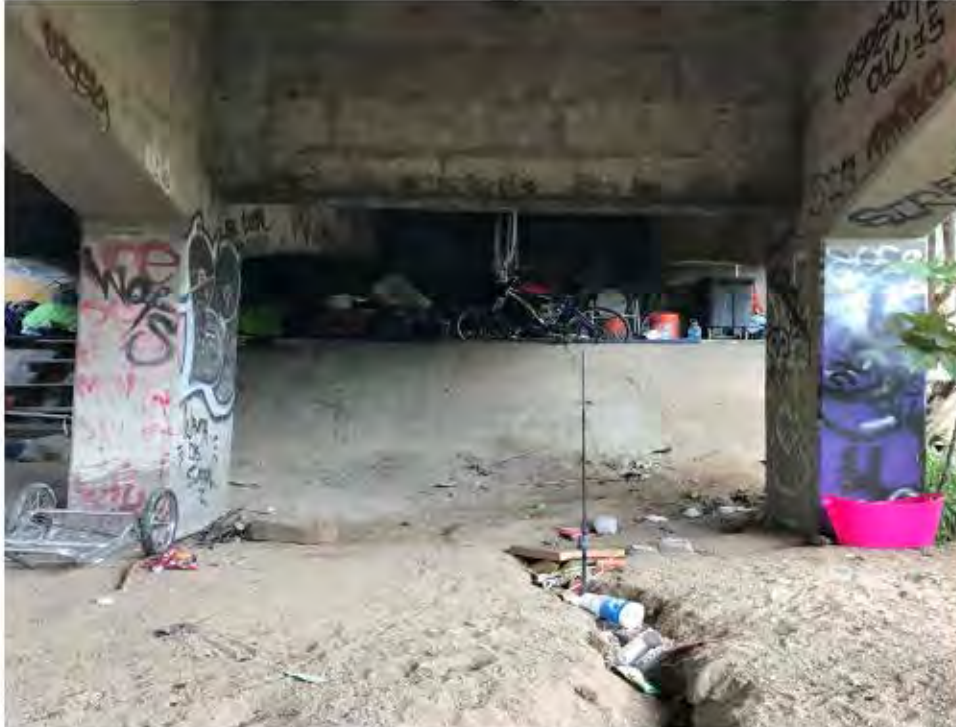
Photo 13: Representative graffiti, Pier 1 facing north (XRF Samples: 047 and 048).
