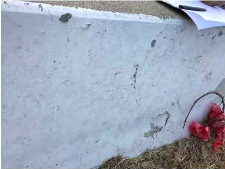
Photo 05: White paint covering graffiti, East Guardrail (Bulk Sample PB-01, XRF Sample 004).
