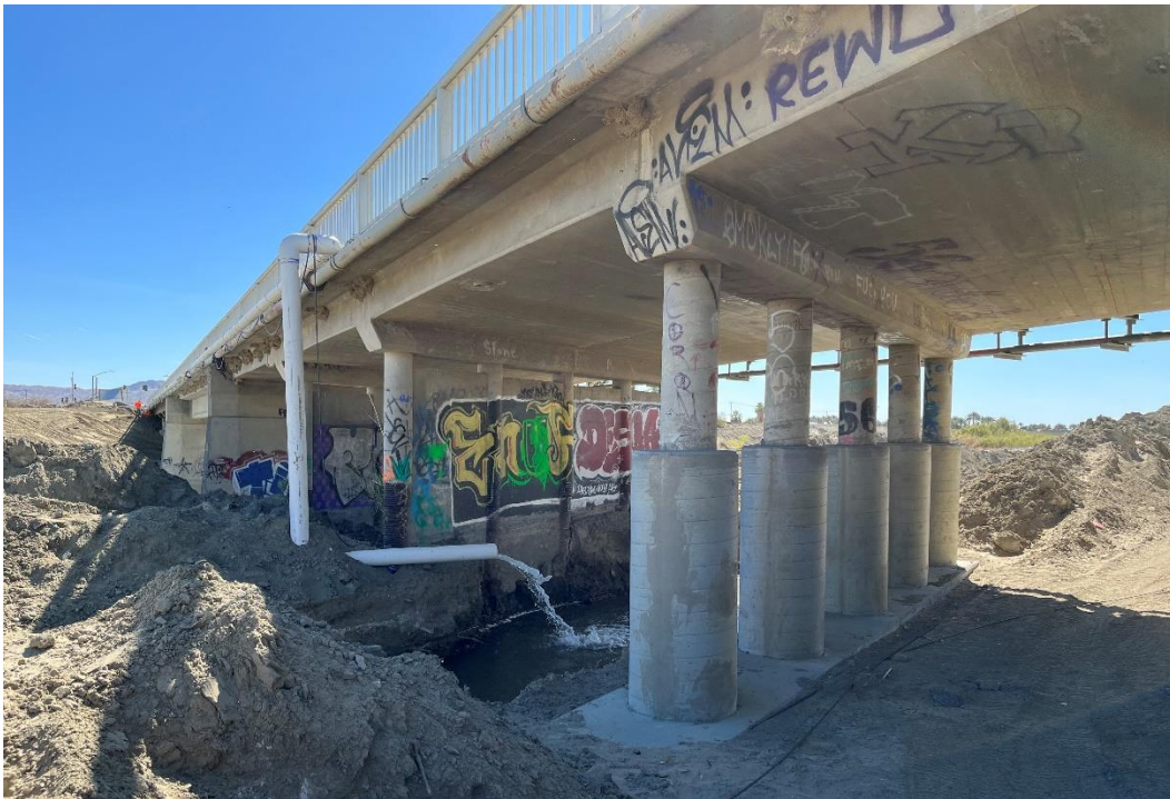
View of Airport Boulevard Bridge columns and exposed footings (March 2022). Photo facing south.
