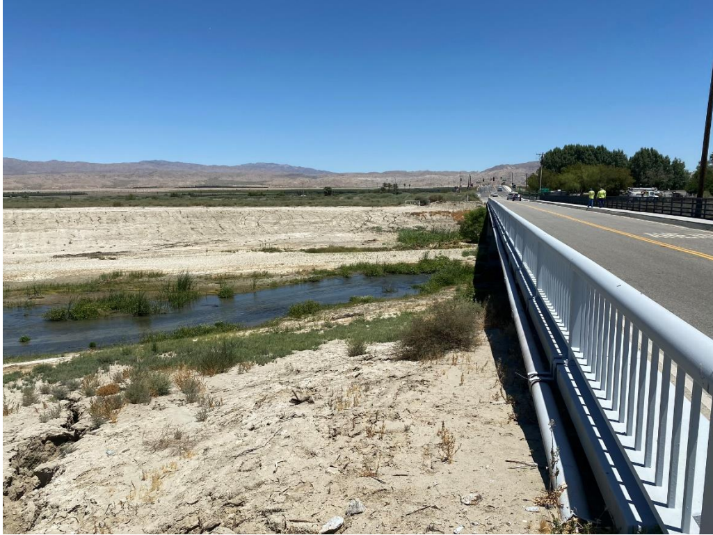
View of Whitewater River facing East showing river channel and utility lines attached to the bridge crossing the river (October 2020).
