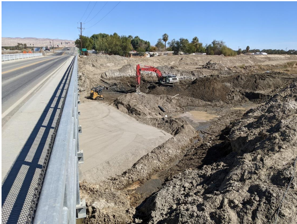
View of Airport Boulevard Bridge and Whitewater River showing recently new yellow striping along Airport Boulevard and new sidewalk and handrail (March 2022). Photo facing east.
