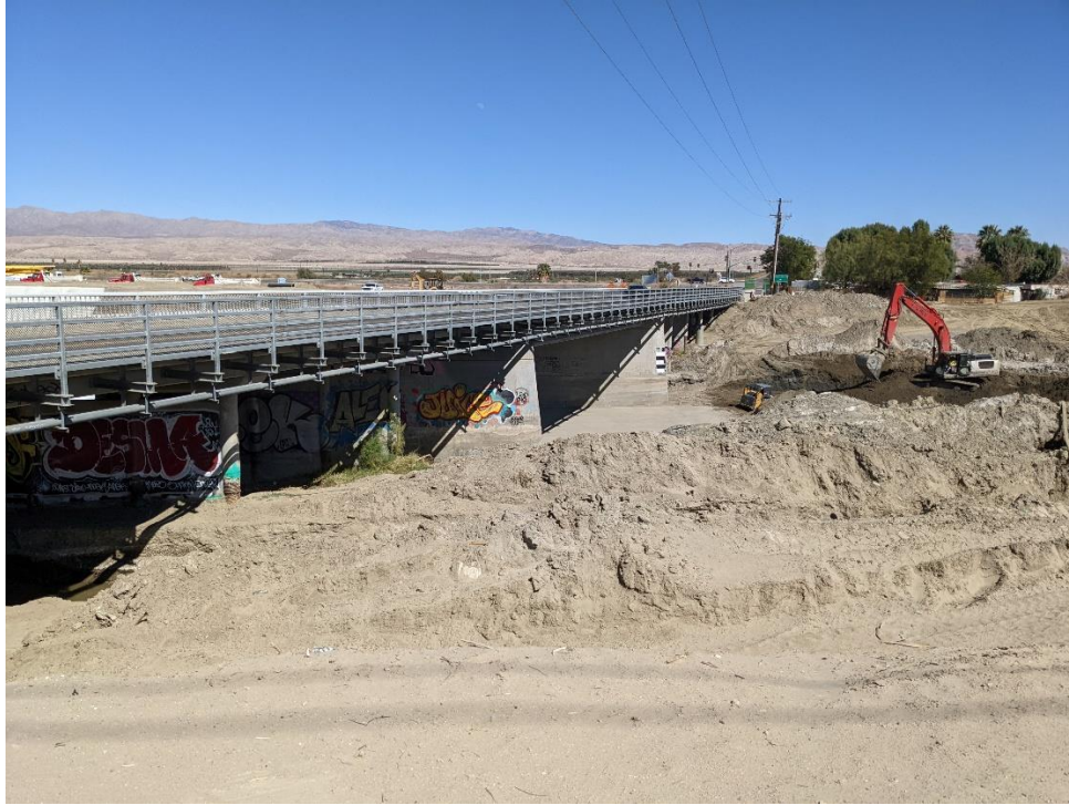
View of Whitewater River, showing CVWD Project currently underway, utility lines attached to the bridge crossing the river, and structural concrete under bridge that may contain asbestos (March 2022). Photo facing northeast.
