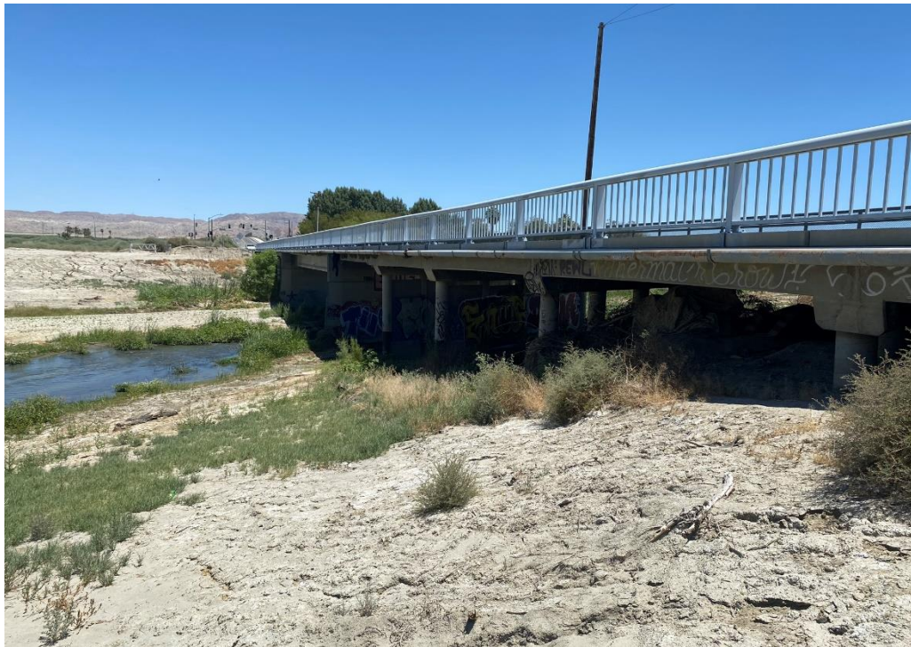
View of Airport Boulevard Bridge over Whitewater River facing East showing structural concrete under bridge that may contain asbestos (October 2020).
