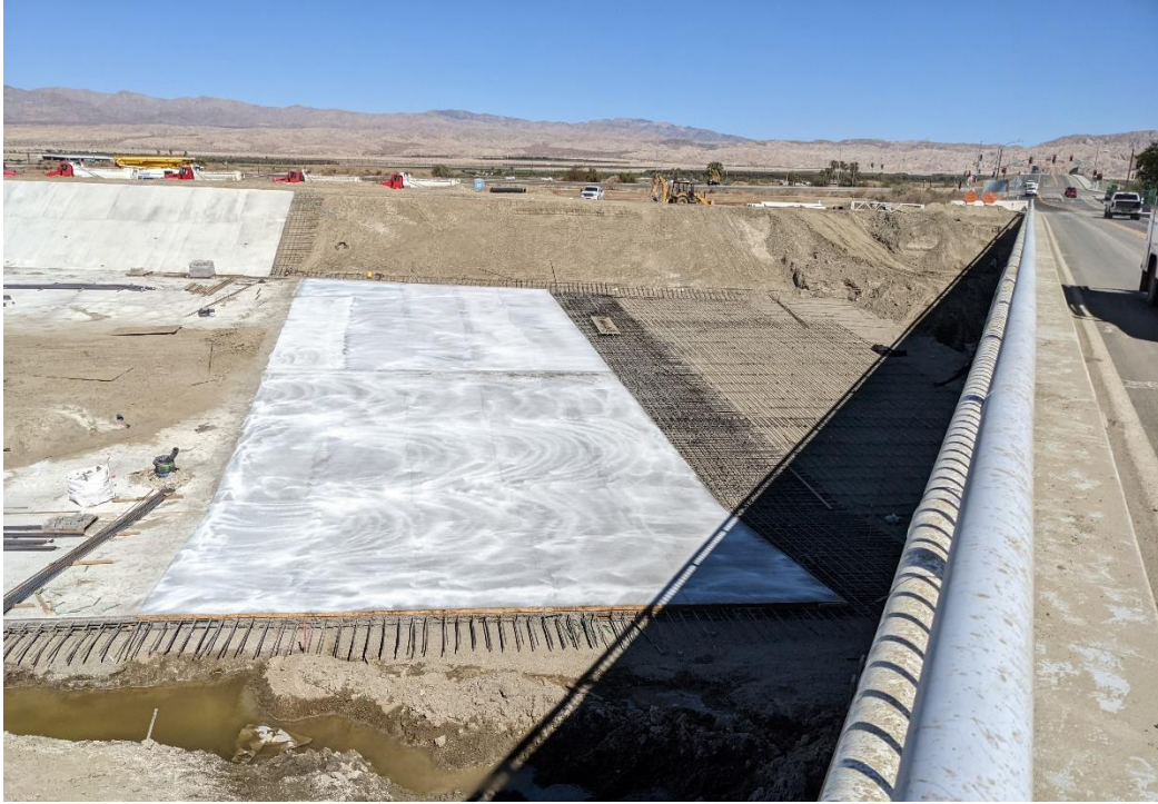
View of Airport Boulevard Bridge and Whitewater River showing new concrete lining under channel (March 2022). Photo facing east.
