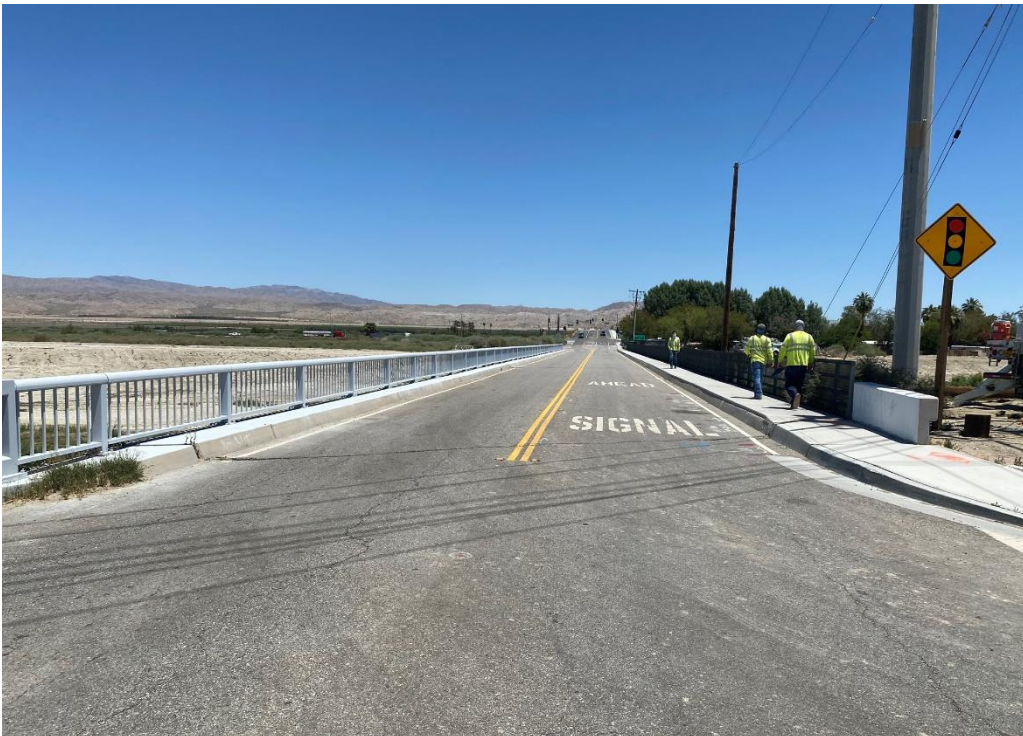
View of Airport Boulevard Bridge facing East showing recently new yellow striping along Airport Boulevard and new sidewalk and handrail on either side of the bridge (October 2020).
