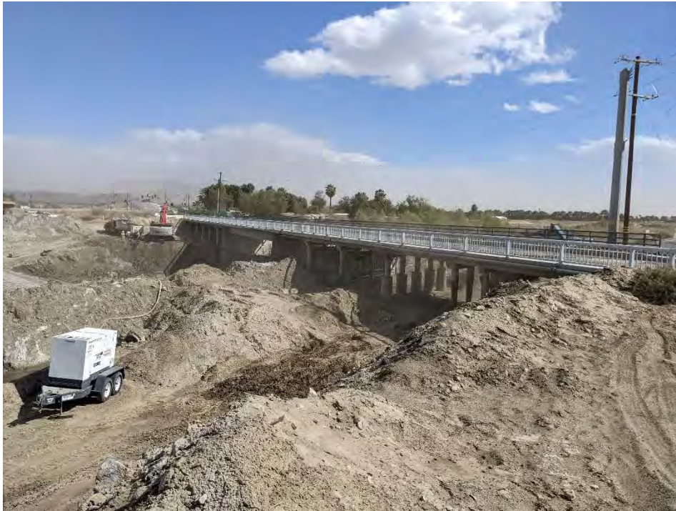
Photo 11. CVWD Stormwater Channel Improvement Project construction lowering the riverbed and replacing Whitewater River with a concrete lined channel at the Airport Boulevard Bridge in March 2022.
