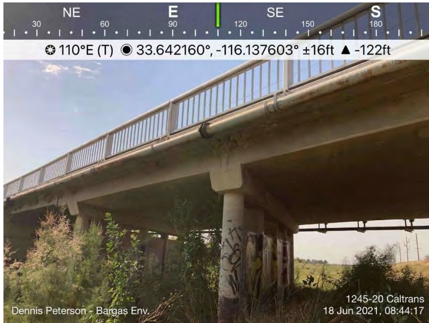
Photo 1. The Common and Giant Reed Marsh plant community within the active channel underneath the Airport Bridge Blvd.
