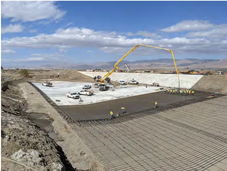
Photo 12. CVWD Stormwater Channel Improvement Project construction lowering the riverbed and replacing Whitewater River with a concrete lined channel at the Airport Boulevard Bridge in March 2022.
